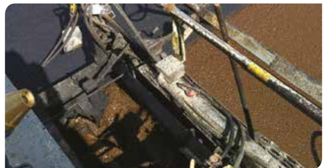
Fresh slurry is brown but cures to a black surface with an appearance similar to hot mix asphalt. Source: Duncor
