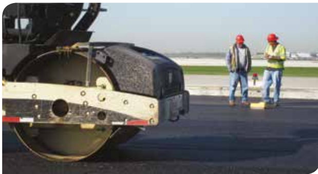
Density measurements being collected from pavement laid using Rediset LQ technology at the O'Hare Airport modernization project.
