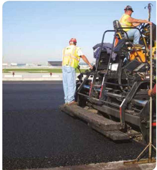
The crew of K-Five Construction Company on their first day of laying Rediset LQ modified pavement at O'Hare Airport.
