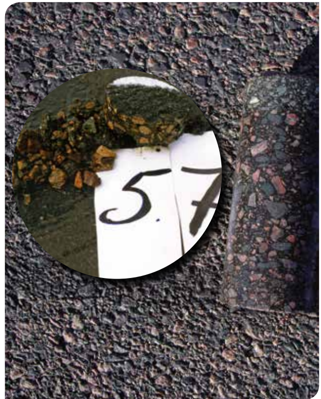
Drilled cores without (left) and with Wetfix liquid adhesion promoters (right) from pavements after twenty years in service..
